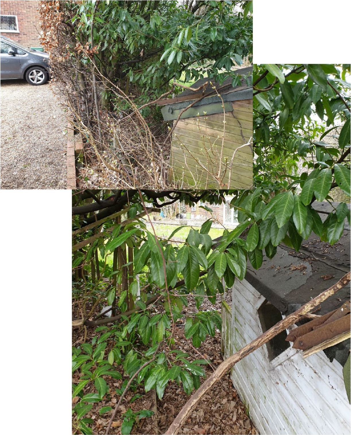
View from 29 Westcote Road showing retaining wall of level car parking area and corner of roof of summer house in garden of 18 Parkside Road
