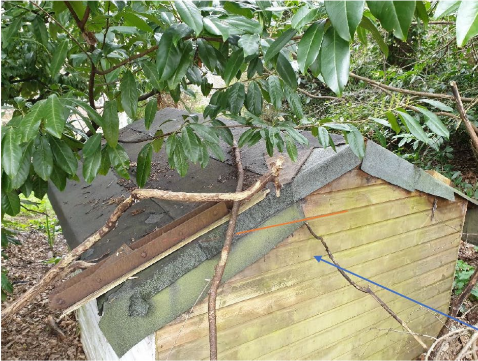
This picture has the laser level line transferred and projected from top of the fence along the boundary between 18 Parkside Road and 16 Parkside Road shown projected onto the back of the summer house.
